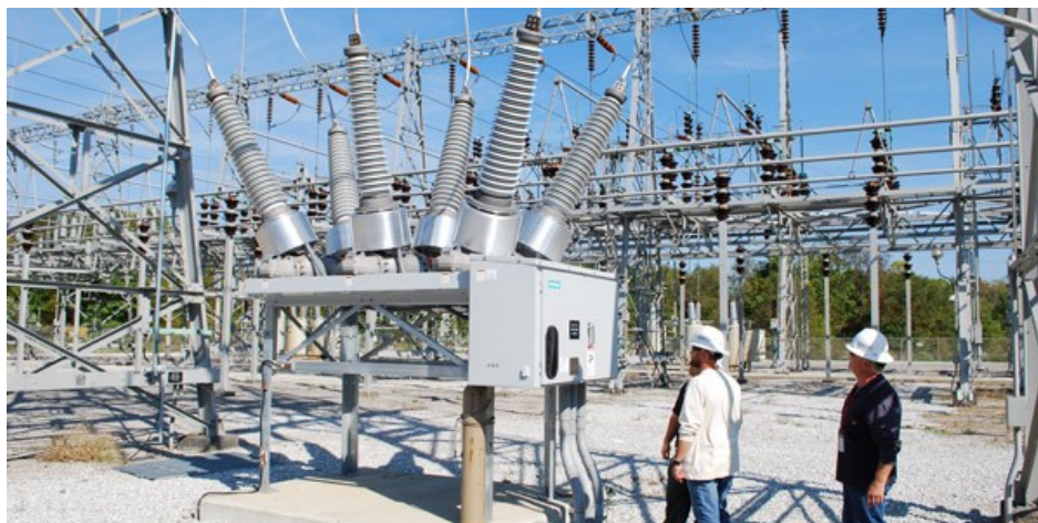
Ohio Edison switchyard | FirstEnergy
